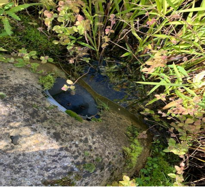
Outlet pipe from Pond A, high level, this pipe sets the water level in Pond A.
