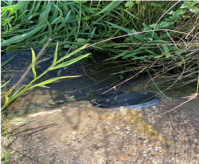
Inlet pipe to Pond B, high level, running clear, bottom photo shows the outlet pipe from Pond B, low level, just visible below water level.
