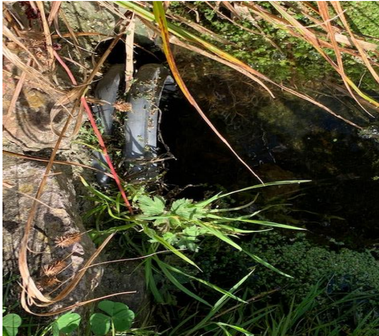
the inlet pipe to Pond D
